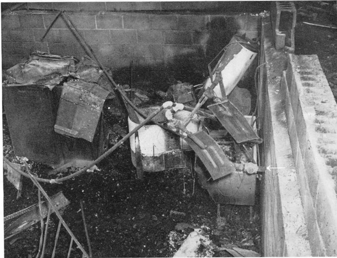
FIG. 16. Remains of foundation of a destroyed home. Note water heater in corner, damaged meter and service shut-off cock on the right (note arrow).
