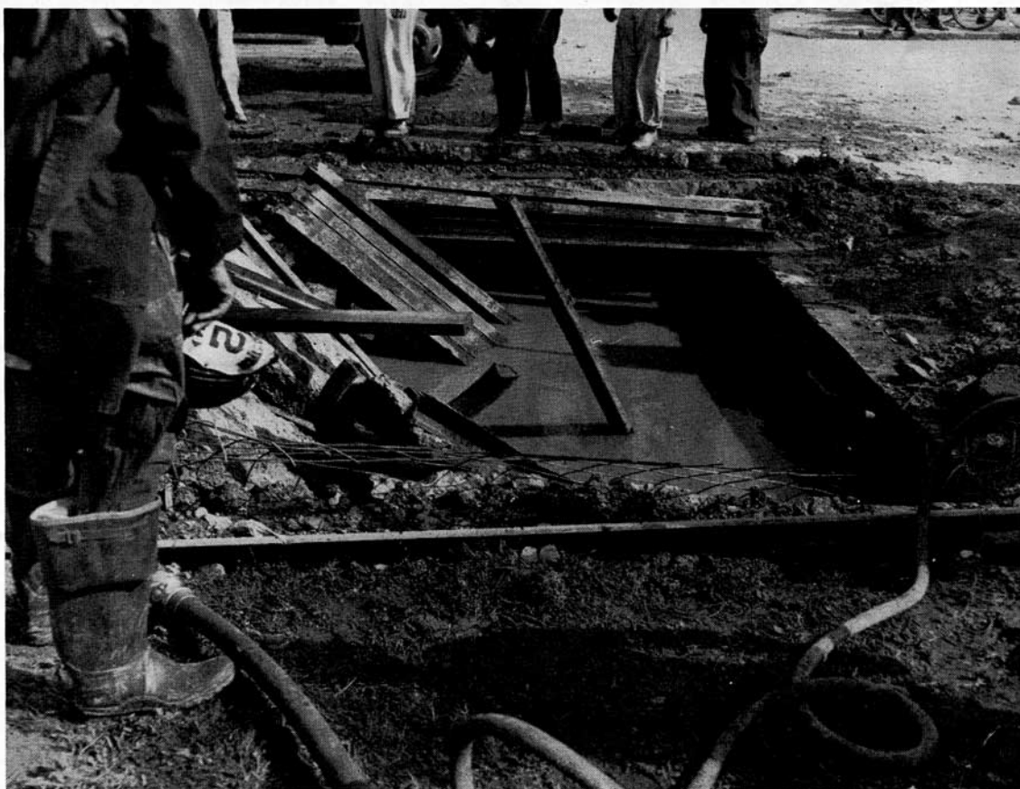
FIG. 5. View of low-pressure regulator chamber after flooding and extinction of flame, showing steel rail reinforcement of damaged roof. Note wire netting and sidewalk construction forms in foreground.
