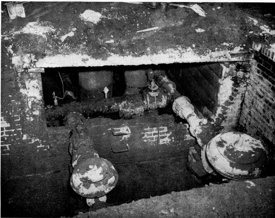
FIG. 7. Interior of regulator vault. Low-pressure regulators in foreground; fogging tank and cross-connection to medium-pressure system in adjacent vault.
