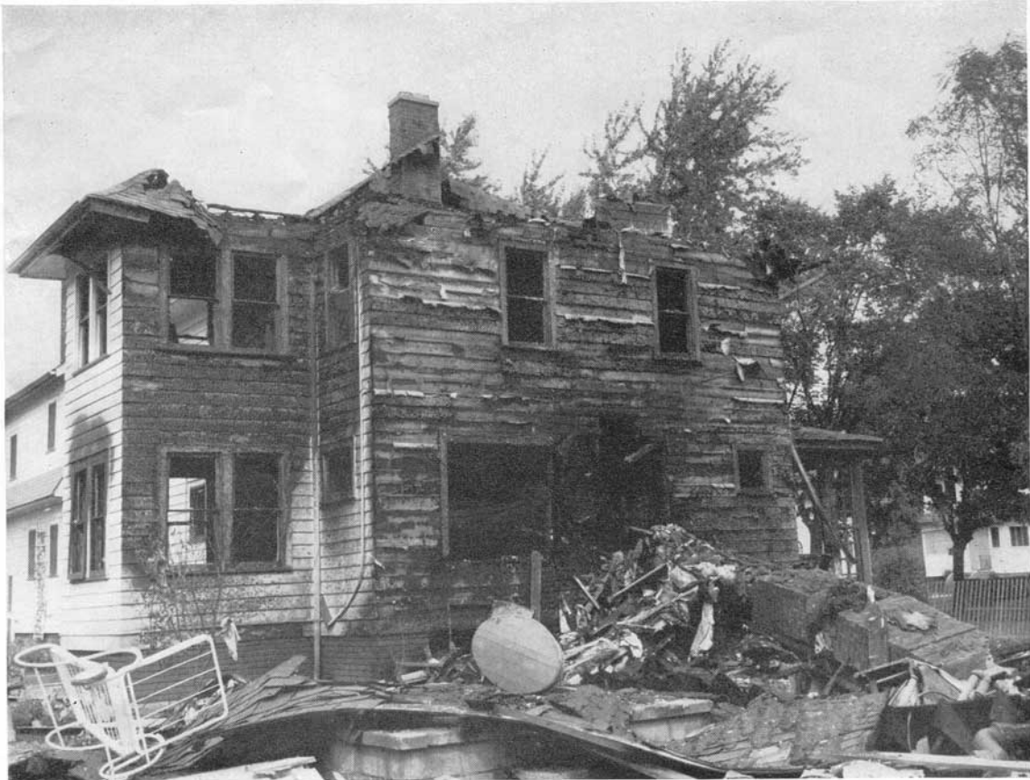
FIG. 18. Exposure fires were frequently severe as this photo taken at Fair Oaks Avenue shows.
